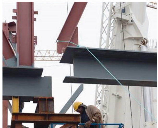
Fig. 30 Detail of the beam of the main building’s external wall under construction
