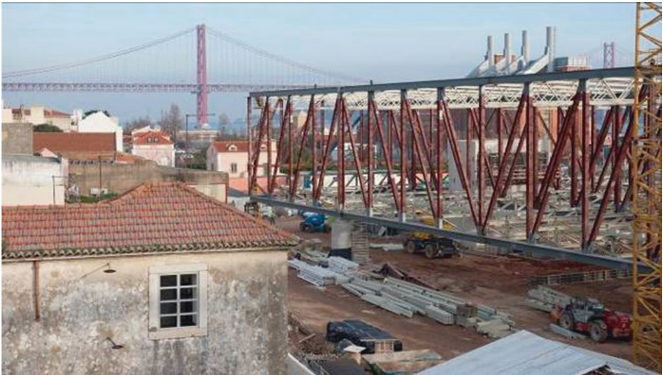
Fig. 24 View of the main building under structural construction phase from the second level of the auditorium
