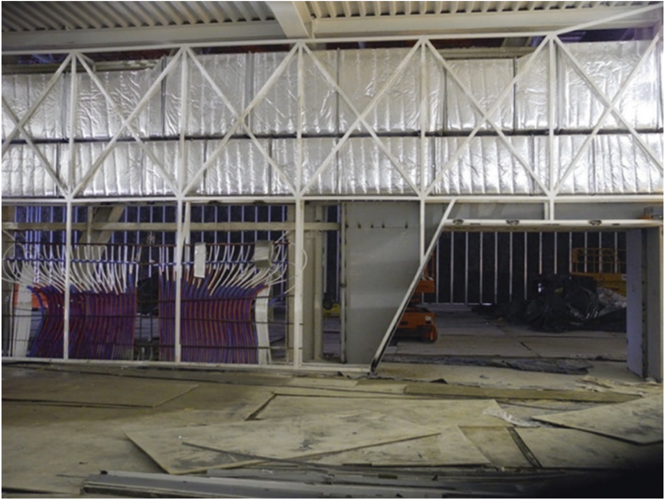
Fig. 90 Ventilation system inside the main wall
